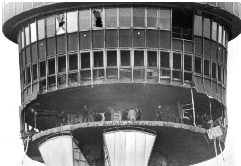
An IRA bomb damaged the tower in 1971, leading to the restaurant's closure
